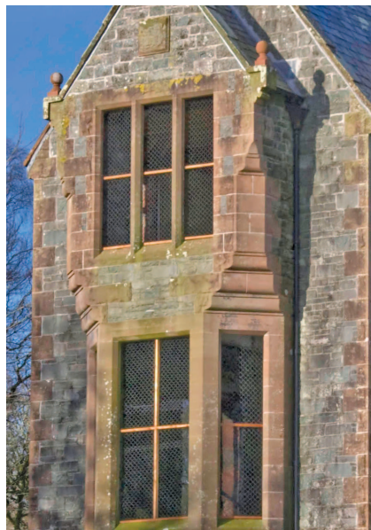
Figure 7. Detail of Maxwell's bedroom windows (second floor) and main living area windows.
